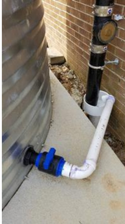
Image 5: Stormwater drain for rainwater collection tank overflow
